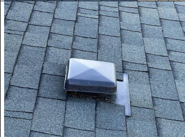
Photograph 96: Closer view of the roof vent shown in Photograph 95.
