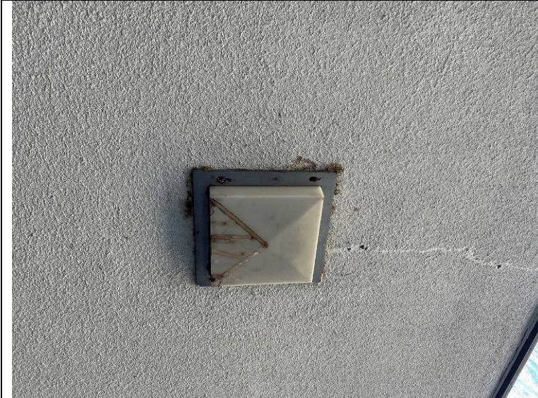
Photograph 5: Water staining at a light fixture in the soffit under the area where test openings were made.
