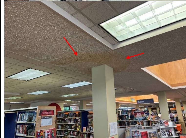
Photograph 54: Area below the area circled in Photograph 51. Arrows indicate apparent water staining on the ceiling.
