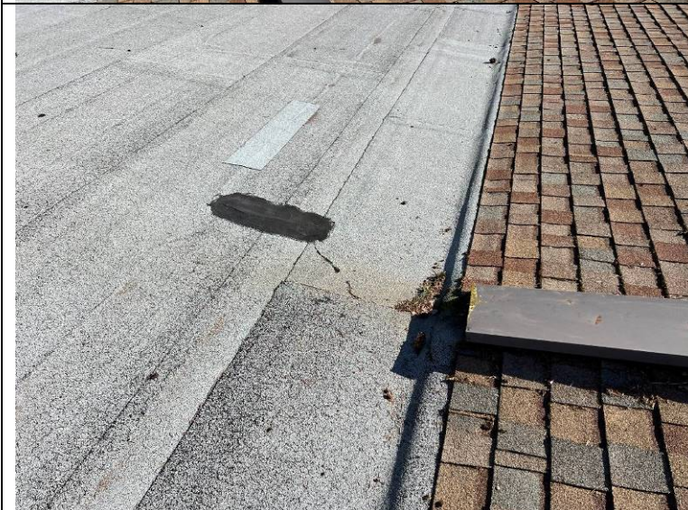
Photograph 78: Closer view of the roof cement patch circled in Photograph 77.
