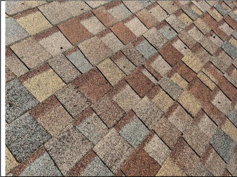
Photograph 61: At the south sloping roofs, the mineral granules are eroding from the surface of the shingles.
