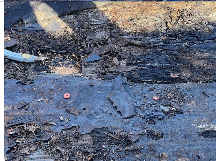
Photograph 12: Closer view of the area shown in Photograph 11.
