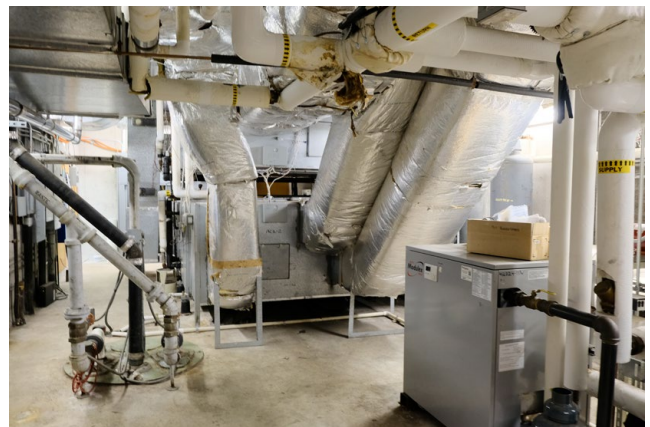
Basement mechanical room
