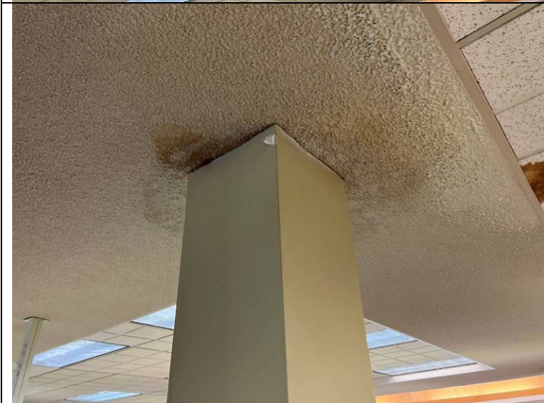
Photograph 81: Closer view of the stained ceiling in the general area shown in Photograph 79.
