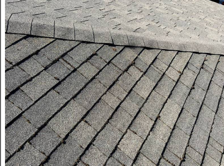
Photograph 89: Moss growth along the perimeter of the shingles.
