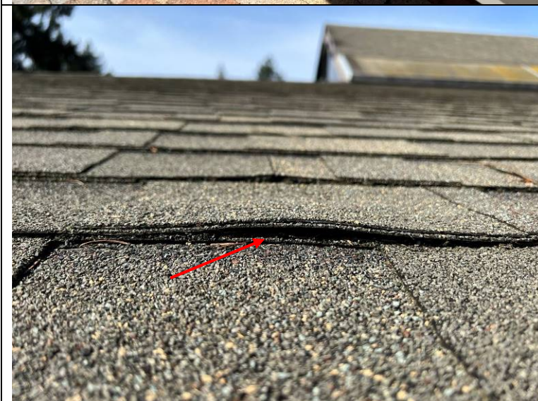
Photograph 105: Arrow indicates an apparent nail backing out and lifting the overlying shingle.
