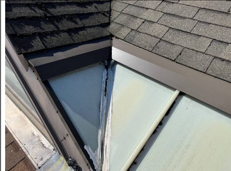
Photograph 53: Sealant at this location is older and was likely applied in response to previous water entry.
