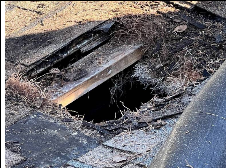
Photograph 19: Closer view of test opening #4 showing the deteriorated cementitious wood fiber substrate board.
