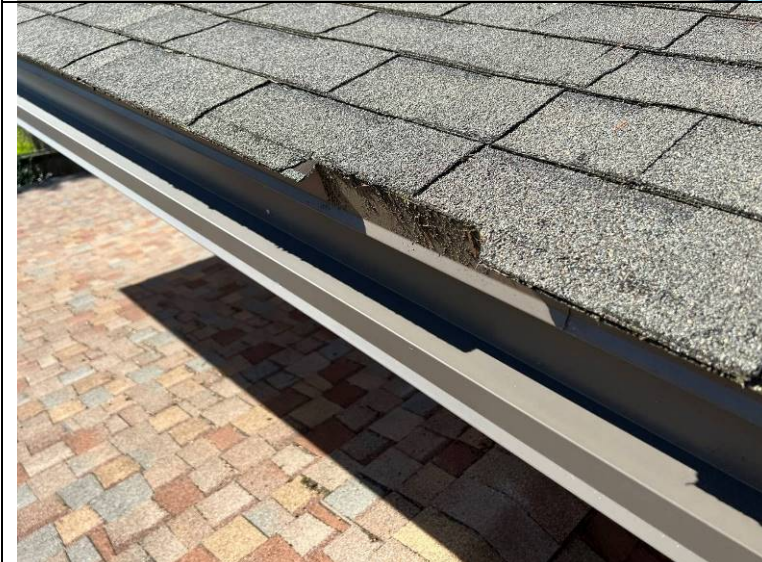
Photograph 104: Damaged shingle at the eave edge.
