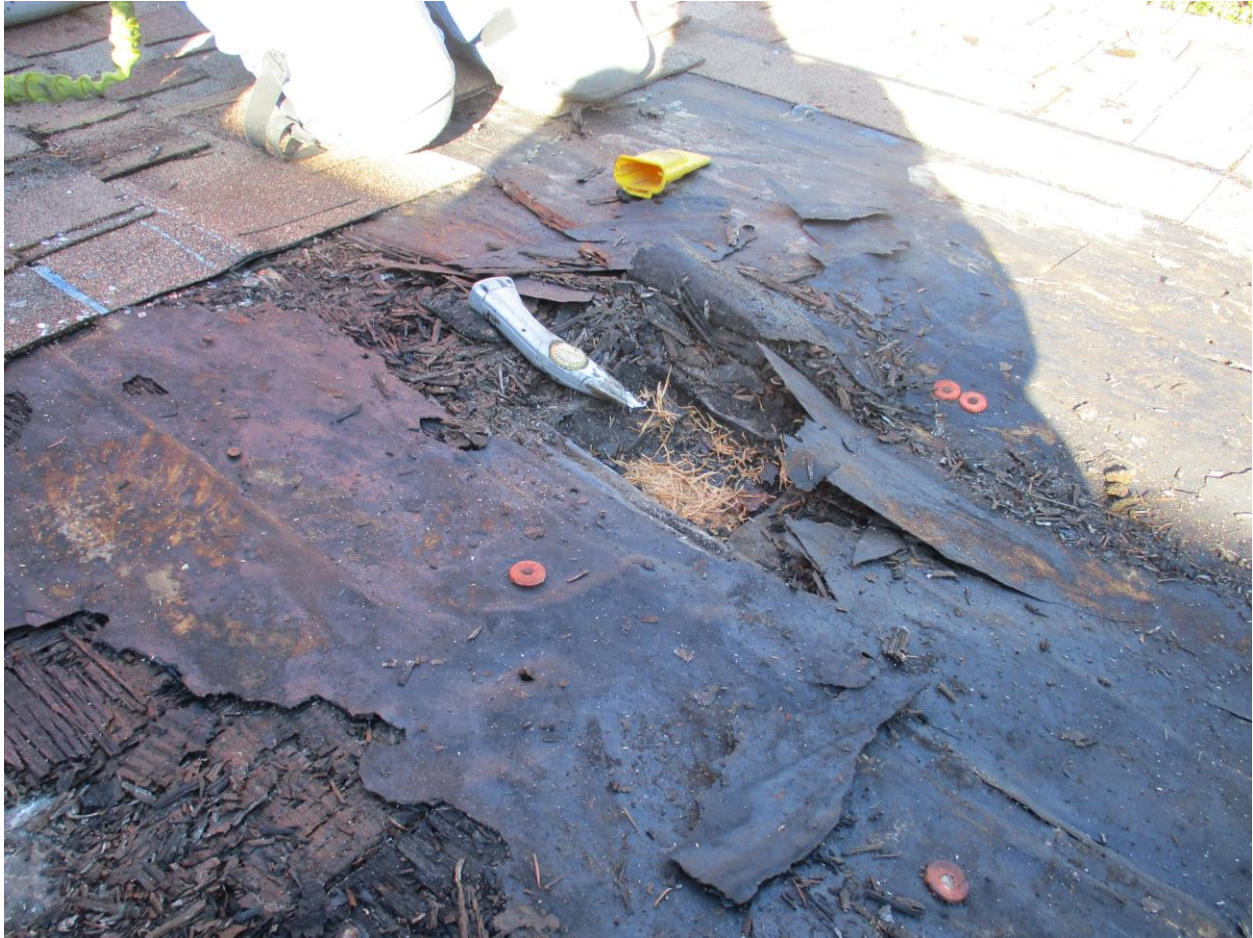
Photo 1 – Deteriorated Plywood Low Roof @ North
