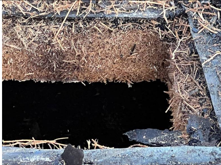
Photograph 14: Closer view of the cementitious wood fiber substrate board at the test opening.
