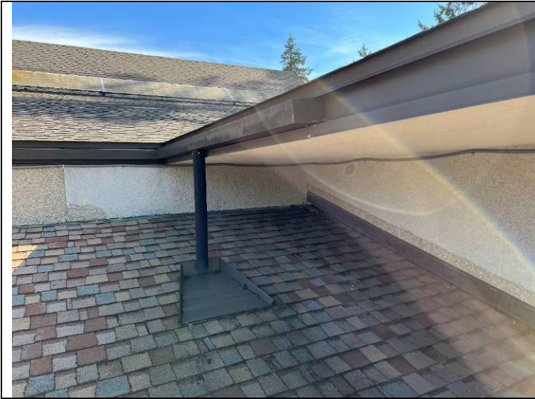
Photograph 100: Downspout and splash pad.
