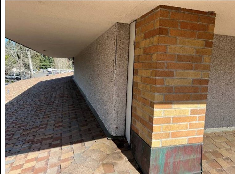
Photograph 35: Cracked marblecrete at a rising wall corner transition.
