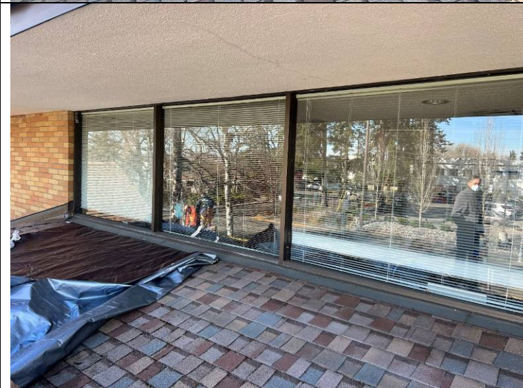
Photograph 27: Windows at the upslope edge of the north sloping roof area. The windows sit less than 5-inches above the surface of the roof.
