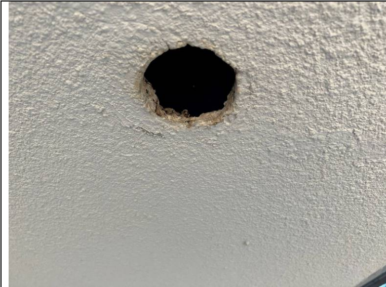
Photograph 103: Closer view of the hole indicated by the arrow in Photograph 102.
