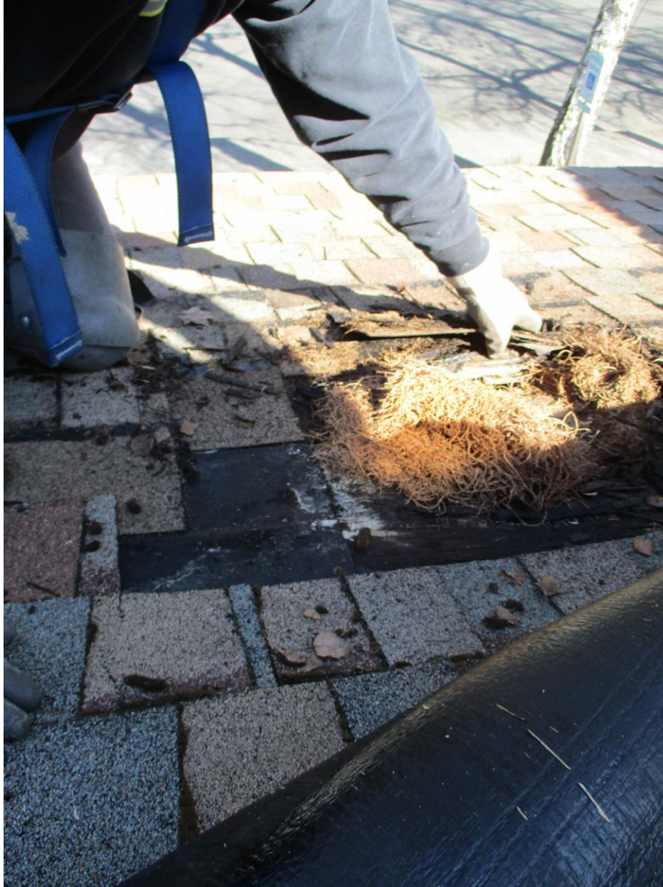
Photo 3 - Tectum Water Damage
