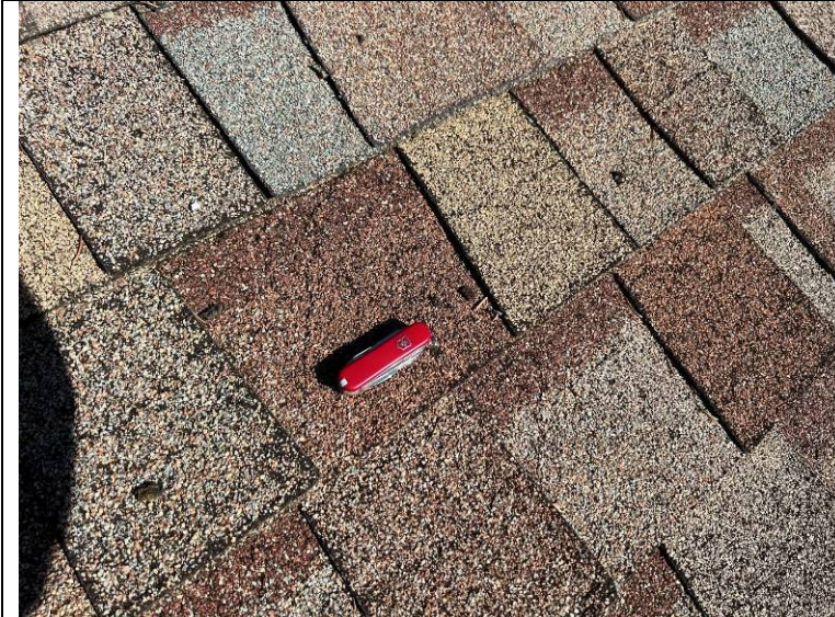
Photograph 62: Closer view of the surface of the shingles.
