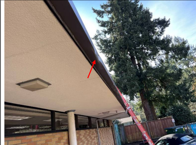
Photograph 68: Damaged gutter (arrow) at the west side of the roof.
