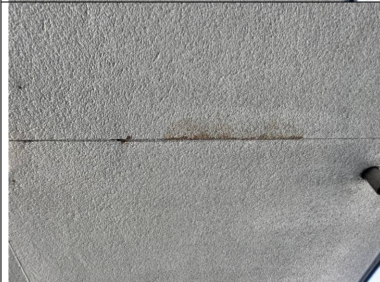
Photograph 6: Water staining at the soffit under the area where test openings were made.
