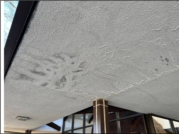
Photograph 4: Water staining at the soffit under the area where test openings were made.
