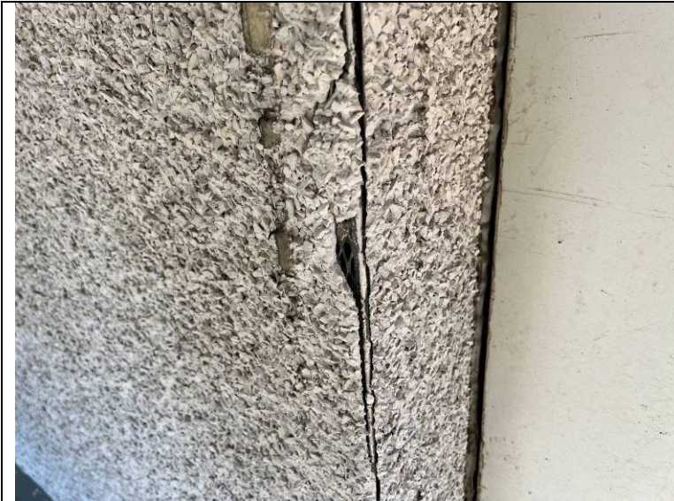
Photograph 37: Closer view of the area shown in Photograph 35. Damage is likely due to age, settling, and differential movement.
