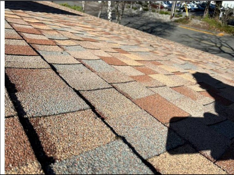
Photograph 25: Slight curling or cupping of the Tamko shingles was observed in various areas of the roof.
