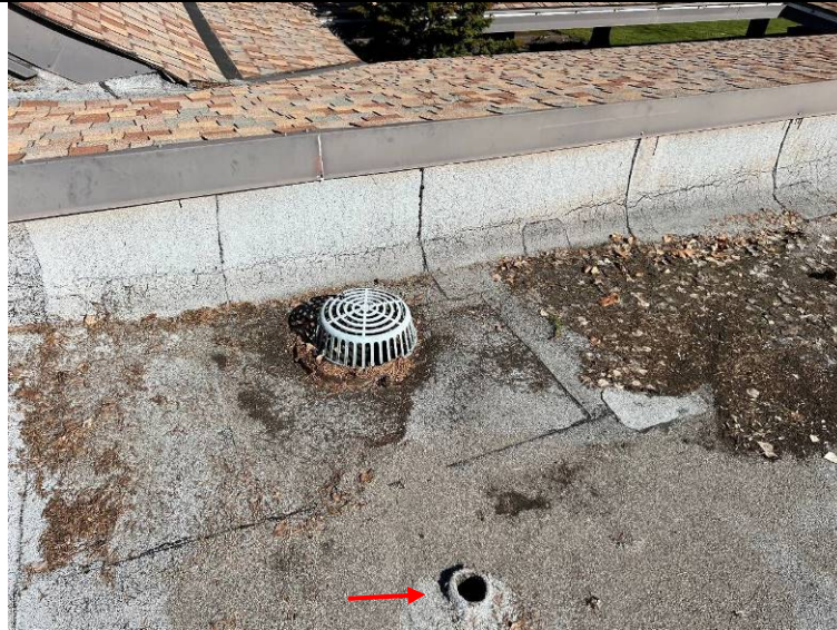
Photograph 75: Closer view of a cast iron roof drain and contractor style overflow (arrow).
