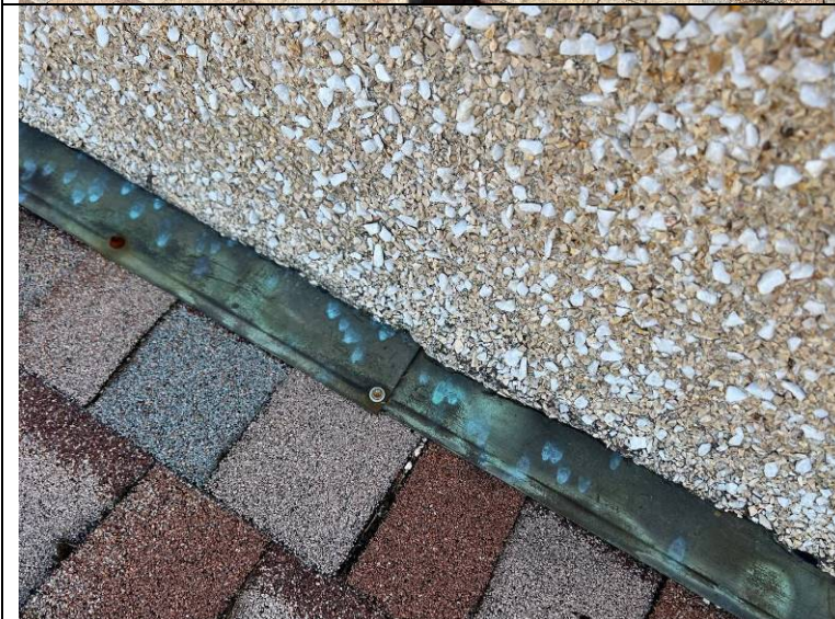
Photograph 33: Closer view of the headwall flashing.
