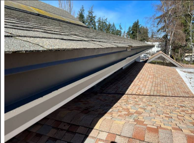
Photograph 101: Eave edge without a gutter.
