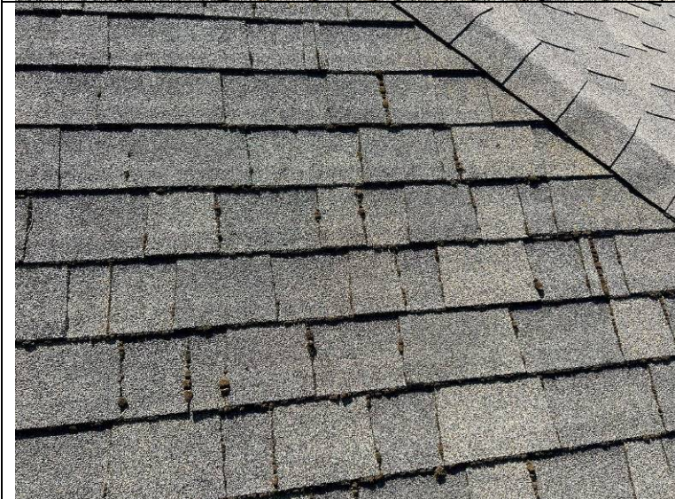
Photograph 90: Alternate view of the moss growth at the upper roof.
