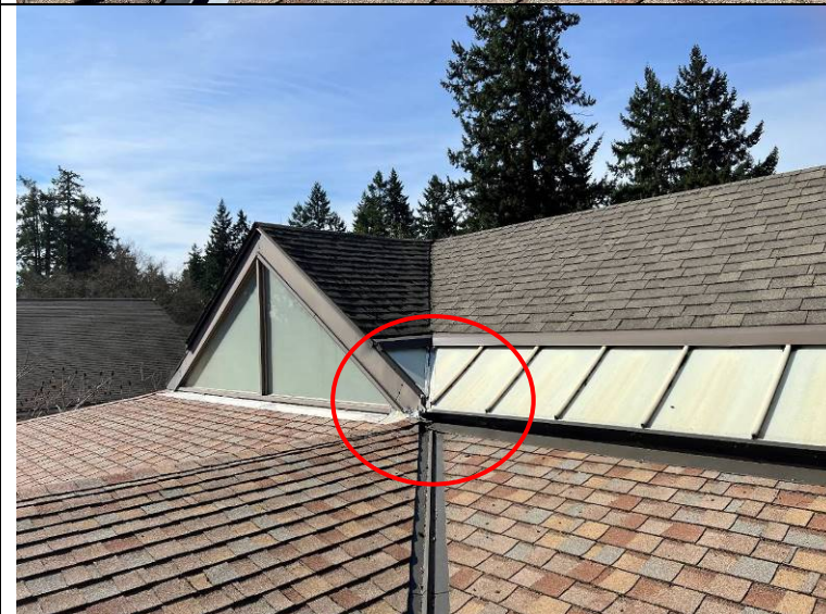
Photograph 51: Overview of a leak location temporarily sealed by Wayne's Roofing.
