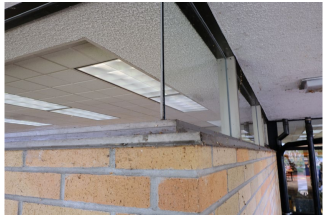
Single pane windows with failed seal at corner joint
