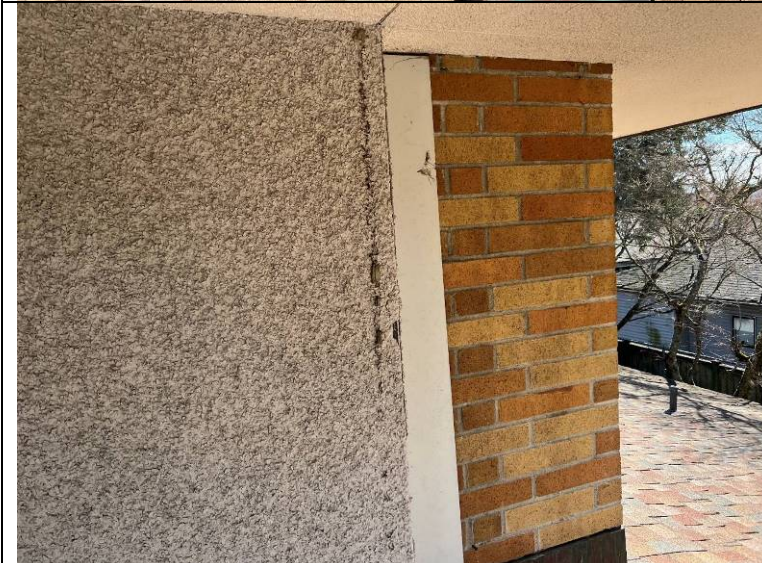
Photograph 36: Closer view of the damage shown in Photograph 35.
