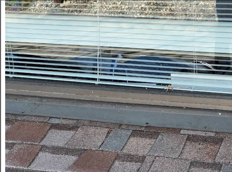
Photograph 29: Closer view of the base of the windows shown in Photograph 27.
