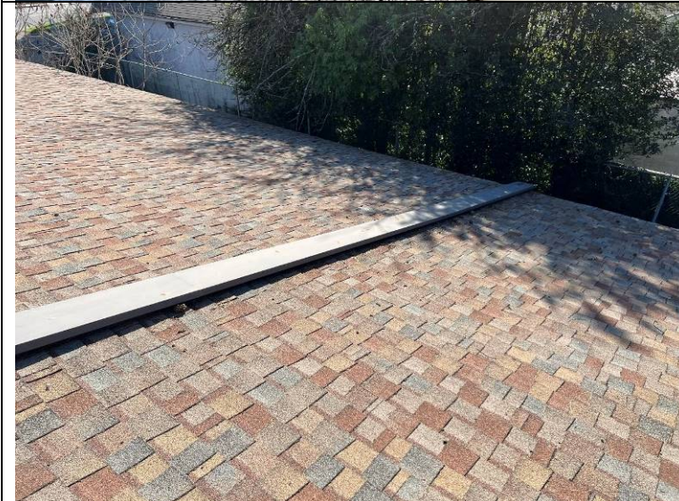
Photograph 38: Sheet metal cover over an area dividing wall. This is situated at the transition between the original building and the 1974 expansion.
