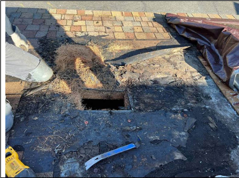
Photograph 13: Portion of the cementitious wood fiber substrate was removed to provide visual access to the structure below.
