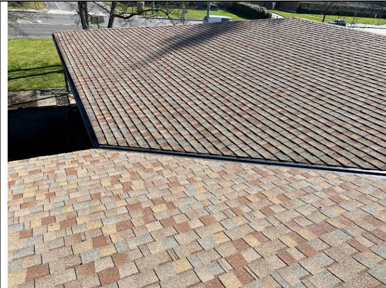
Photograph 49: Typical valley at the lower roofs configured with a sheet metal valley flashing.
