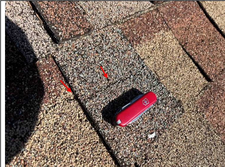
Photograph 64: Cracked shingles at the south sloping roof. (Arrows)
