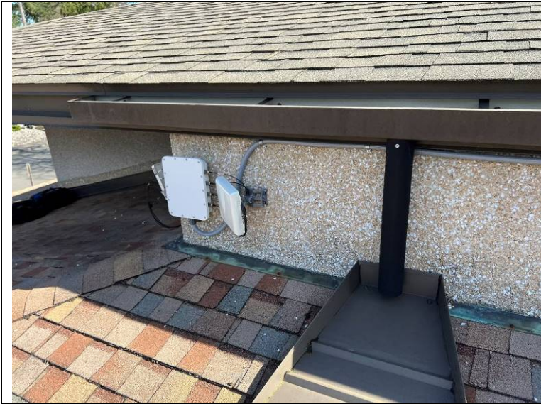
Photograph 67: Equipment mounted to the exterior wall through the marblecrete.
