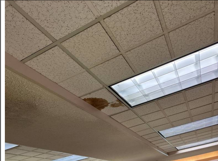
Photograph 80: Closer view of stained ceiling tiles shown in Photograph 79.
