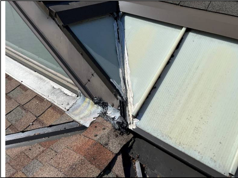
Photograph 52: Closer view of the area shown in Photograph 51. Roof cement appears to have been applied in response to the previous water entry.
