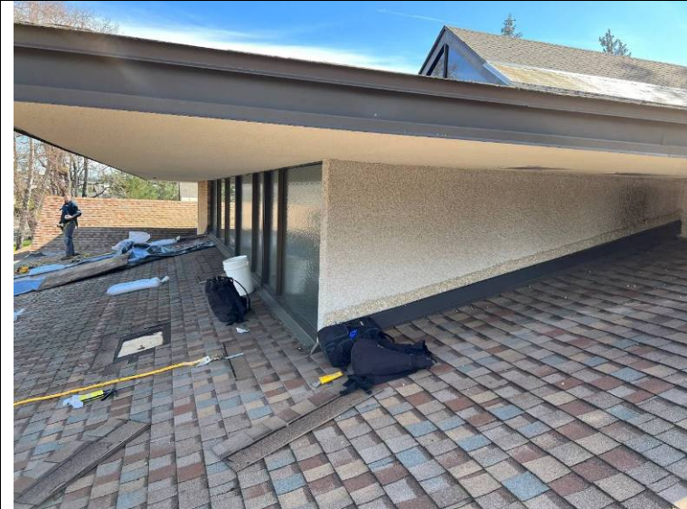
Photograph 26: Looking east along the rising window wall at the north sloping roof area.
