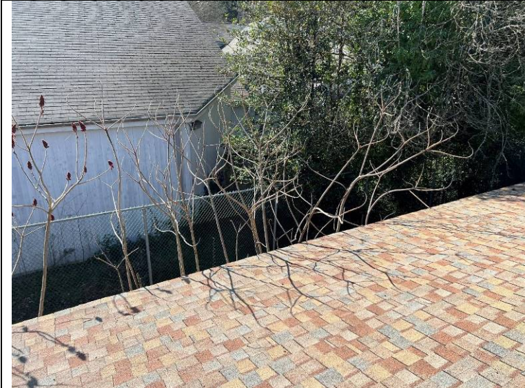
Photograph 59: Trees in close proximity to the roof along the south side of the roof.
