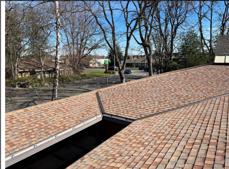
Photograph 44: Opening in the roof at the north central side of the roof.
