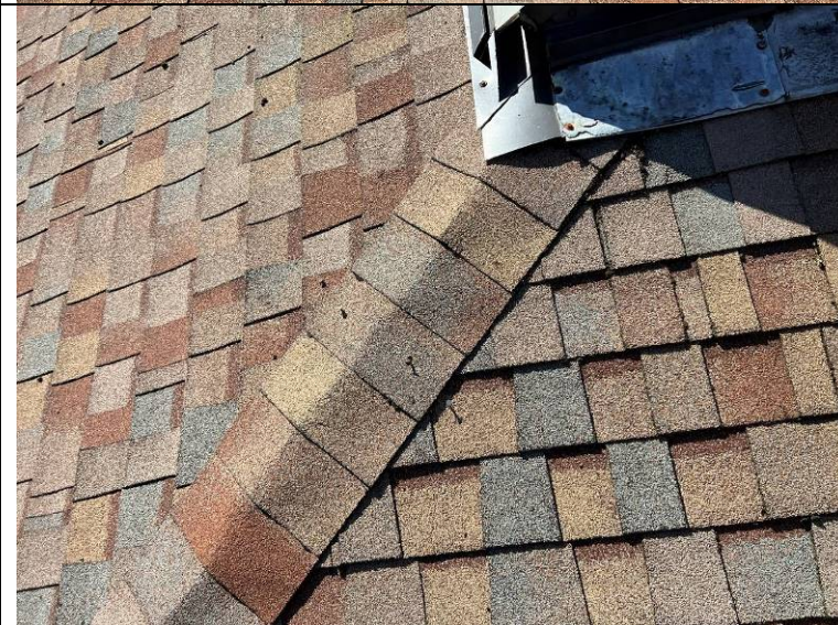
Photograph 47: Closer view of the backed-out nails.
