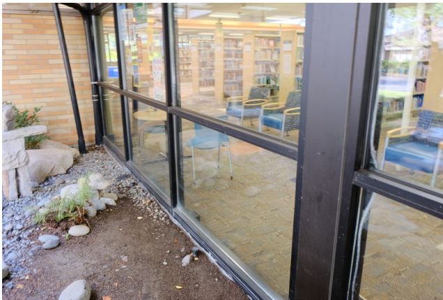
Windows near entry with failed glazing seals
