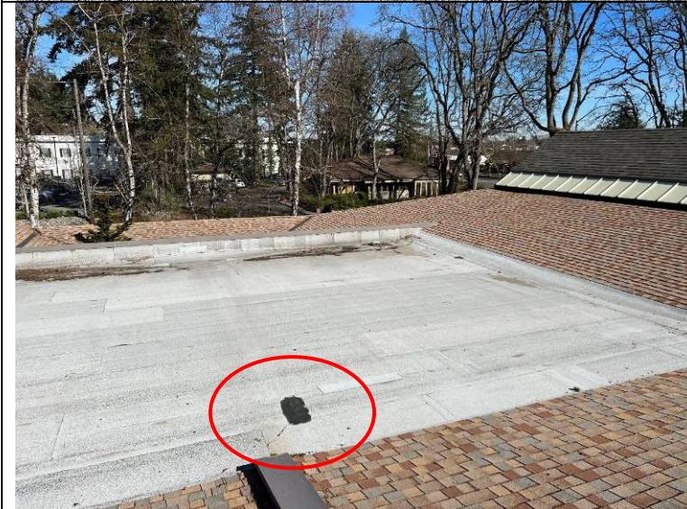
Photograph 77: Roof cement patch over an apparent location of damage.
