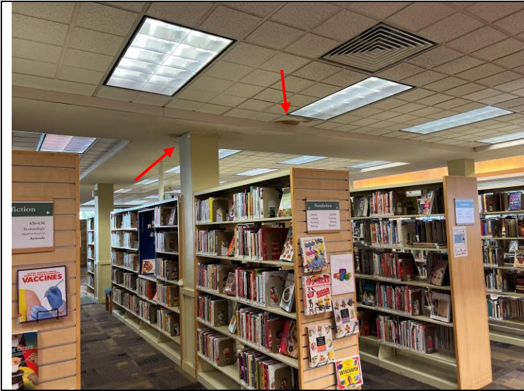
Photograph 79: Approximate area beneath the roof cement patch shown in Photographs 77 and 78.
