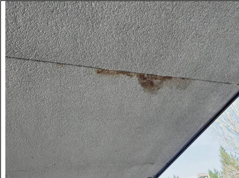
Photograph 7: Water staining at the soffit under the area where test openings were made.
