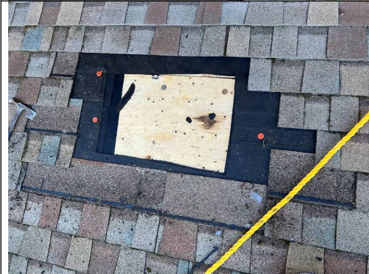
Photograph 8: Test opening #1 was situated under the overhang from the upper roof. The plywood at this location appears light in color and solid.
