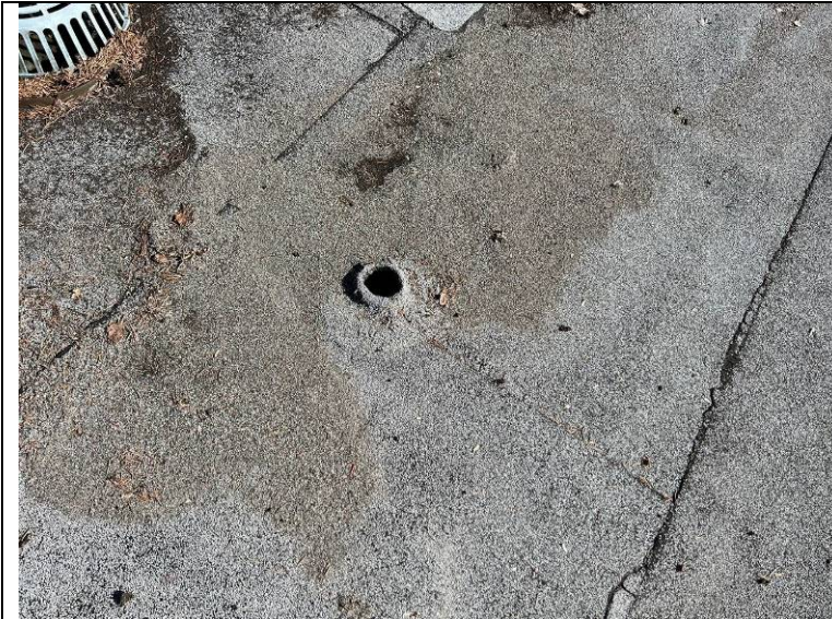
Photograph 76: Closer view of the contractor style overflow.
