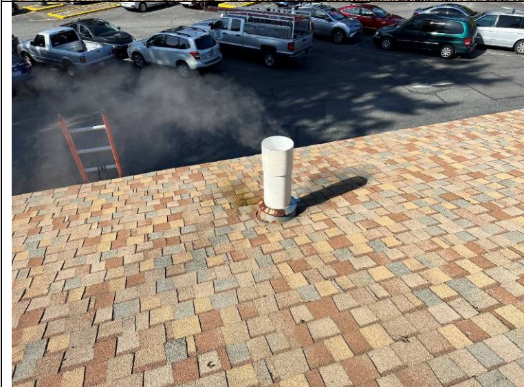
Photograph 65: Boiler vent penetration.
