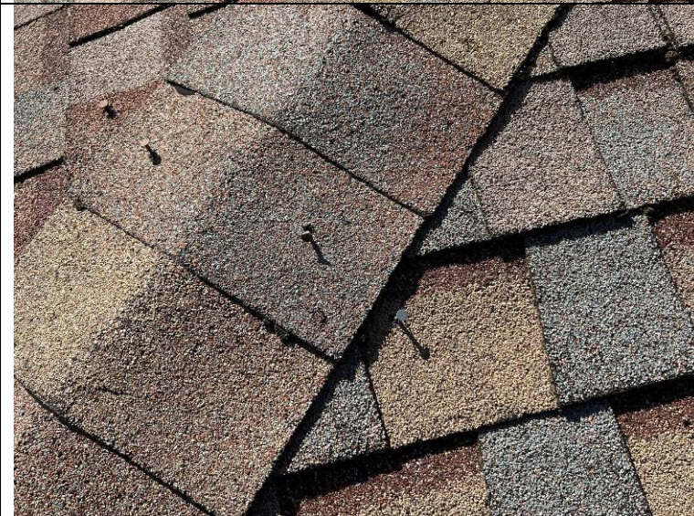
Photograph 48: Closer-up view of the backed-out nails.
