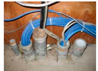
Electrical and data is at capacity at most facilities.
